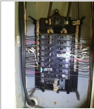
Image of service entrance and branch wires
