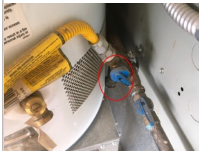
Image of appliance gas shutoff valve.
