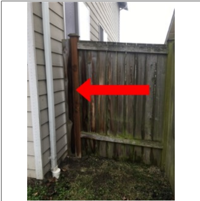
View of fence/fence post on west side of building. The post is slightly loose and I would recommend further monitoring.
