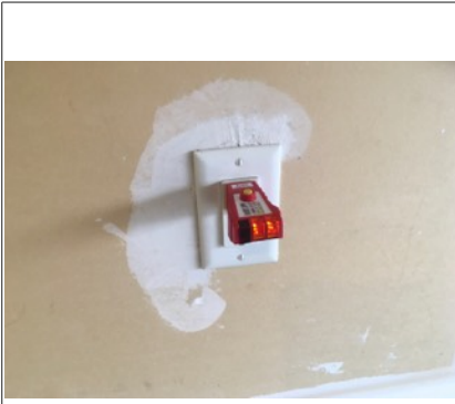
Image of tested GCFI electrical outlet on interior of garage.
