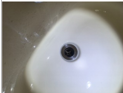
The tub stopper is missing and should be replaced.
