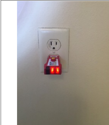
Image of tested electrical outlet
