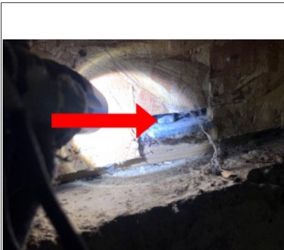
Image of seismic plate and bolt.
