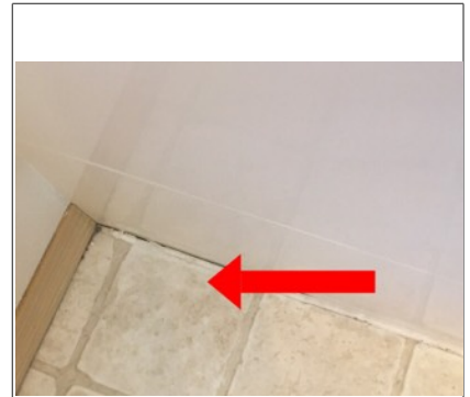
Missing caulking around bottom of shower/tub to prevent water intrusion into flooring.
