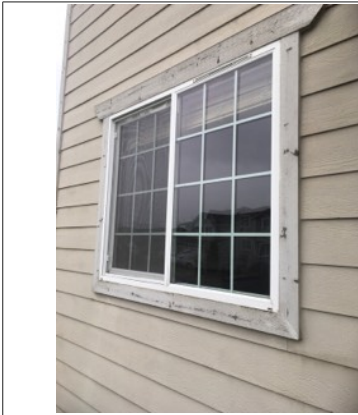
Image of exterior window. All windows are same make/material as picture in this photo.
