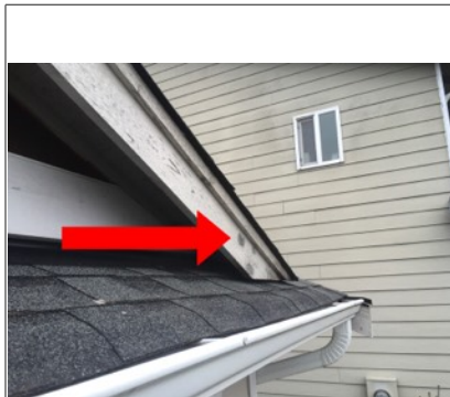
Image of fascia board on front of house. Recommend sealing/painting to reduce water penetration into wood.
