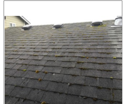
Image of moss/mold build-up on shingles. Roof vents near ridge.
