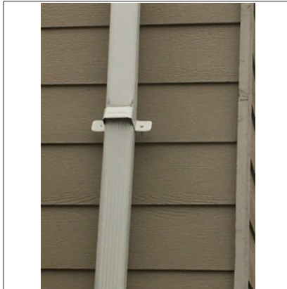
Loose downspout attachment. Recommend further evaluation/repair by licensed contractor.
