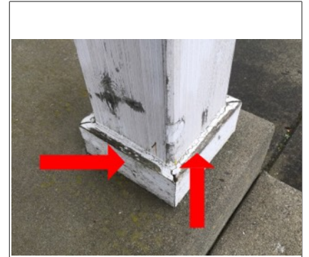
Image of porch cover column. The wood trim on the bottom of the column appears to have moisture intrusion. Recommend sealing and re-painting to prevent further moisture from entering wood.
