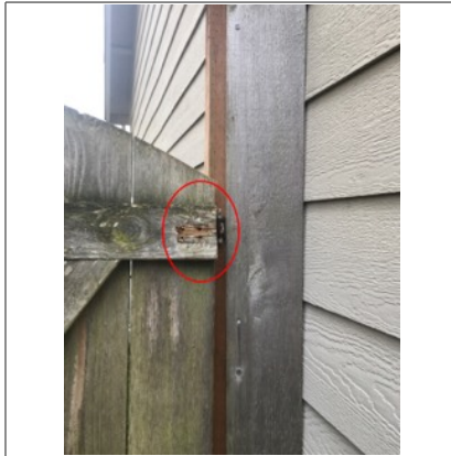
The fence door/gate is missing hardware to lock gate. Recommend repair/replacement by licensed contractor. The fence door binds against the post.
