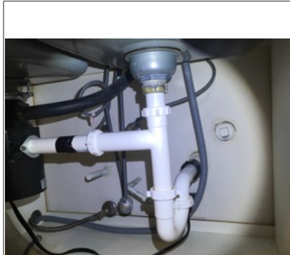
Image of plumbing under kitchen sink.
