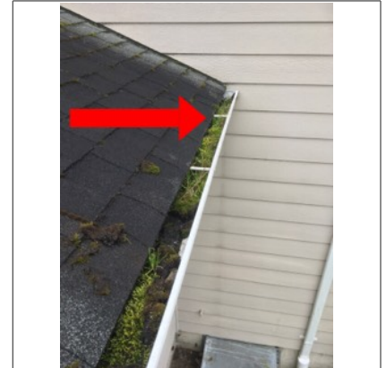
There is build-up in the gutter on the north side of the building. Recommend cleaning out debris.
