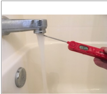
Water is 130 degrees out of 2nd bathroom tub. This could be a SAFETY ISSUE and recommend adjustment of temperature setting on hot water tank. If temperature cannot be adjusted properly I would recommend further evaluation/repair by licensed plumbing contractor.
