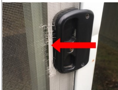
Image of damage to screen on sliding glass door. Recommend further evaluation/repair by licensed contractor.
