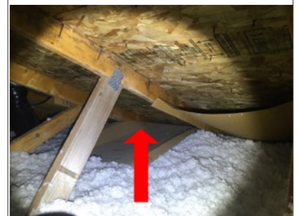
Several insulation baffles have come loose from the trusses. Recommend reattaching baffles to roof trusses.
