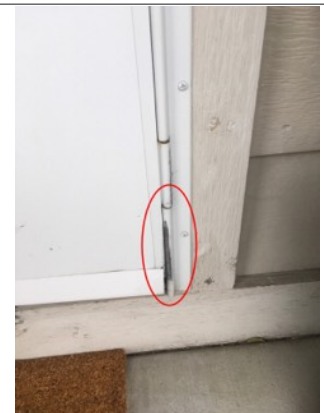
There appears to be rubbing around the hinge on the entryway storm door. Recommend further monitoring.
