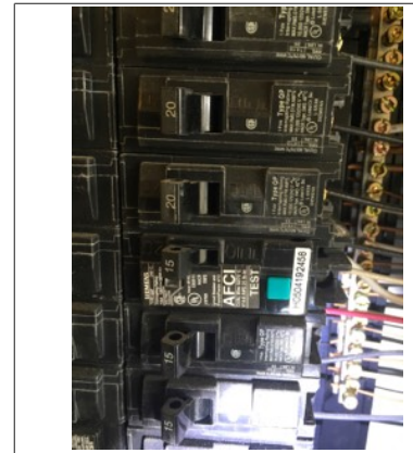
Image of AFCI breakers (two of them inside panel)
