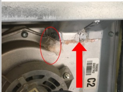
There appears to be mineral residue next to the draft inside HVAC unit. Recommend further evaluation by licensed HVAC contractor.
