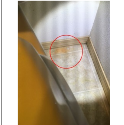
Image of stains on floor. No active water leak present.
