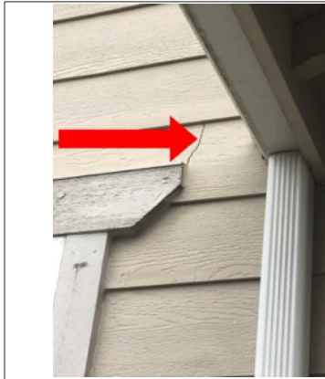
There is a crack in the siding above the window located on right side of the front of structure. This crack could be allowing water/moisture to enter the wall envelope. Recommend further evaluation/repair by licensed contractor.
