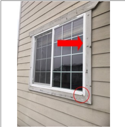
Check caulking around windows and doors along this edge.
