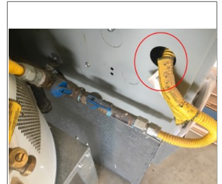
Flexible appliances connectors should not enter appliance cabinet. This could be a SAFETY ISSUE and recommend further evaluation/repair by licensed plumbing contractor.
