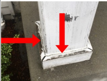
Image of porch cover column. The wood trim on the bottom of the column appears to have moisture intrusion. Recommend sealing and re-painting to prevent further moisture from entering wood.
