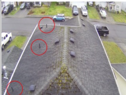
Image of plumbing vents on roof
