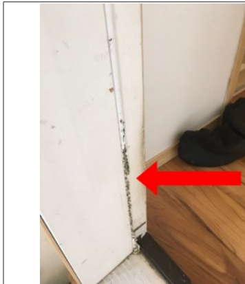
Damaged weatherstripping on garage door (into house). Recommend further evaluation/repair by licensed contractor.
