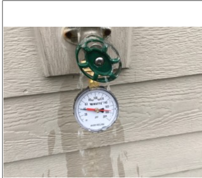
Image of water running from back of house hose bib.
