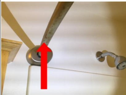
Rust evident on shower curtain rod.
