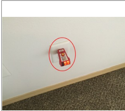
Image of tested electrical outlet
