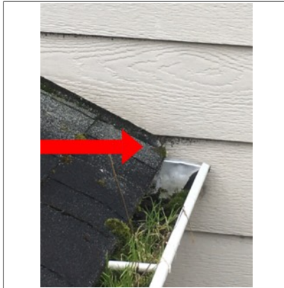
Missing kick out roof flashing. Recommend further evaluation/repair by licensed roofing contractor.
