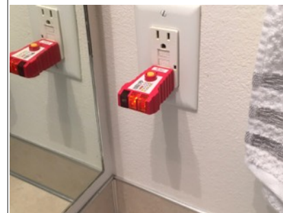
Image of tested GCFI outlet in second bathroom. This GCFI outlet controls all three bathroom receptacles.
