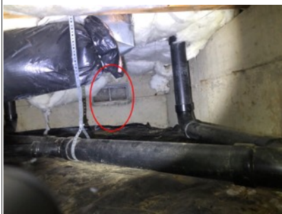
Crawl space ventilation covered/sealed on northeast corner of building. Recommend further evaluation by licensed contractor.
