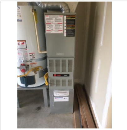
Image of HVAC unit in garage
