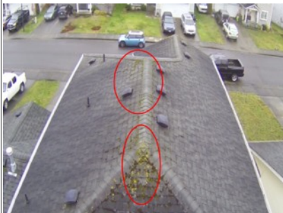
Moss/Mold build-up on roofing materials. Recommend further evaluation/repair by licensed roofing contractor.
