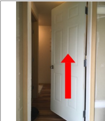
The garage door does not automatically/properly close. This could be a SAFETY ISSUE and should be evaluated/repared by licensed contractor.
