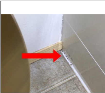
Missing caulking around bottom of shower/tub to prevent water intrusion into flooring.
