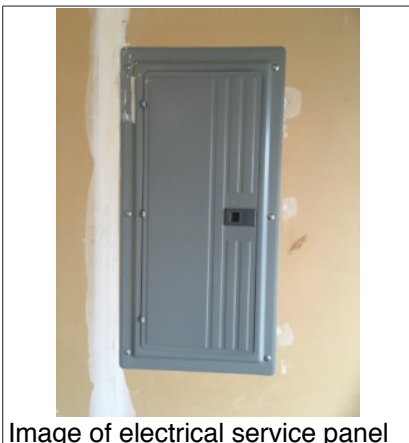
Image of electrical service panel
