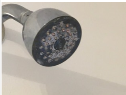
Image of build-up on shower head. Recommend cleaning/replacement if necessary.
