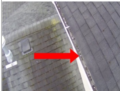
Asphalt shingle granules evident in gutter system.
