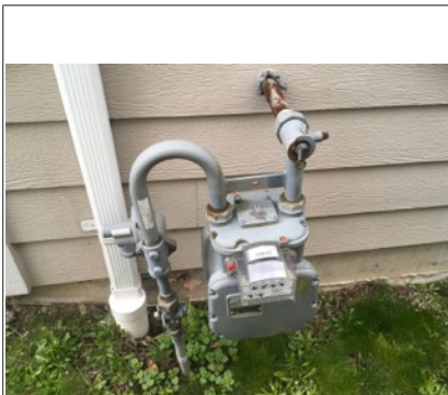
Image of gas meter on east side of building
