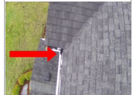
Asphalt shingle granules evident in gutter system.
