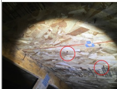
Roofing nails slightly rusty inside attic. Recommend further monitoring for possible issues with ventilation.
