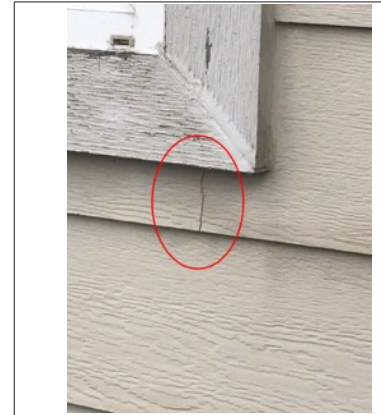
There is a crack in the siding below the window located on right side of the front of structure. This crack could be allowing water/moisture to enter the wall envelope. Recommend further evaluation/repair by licensed contractor.
