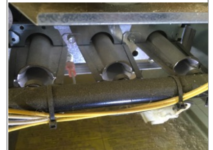
Image of burner ports on HVAC unit
