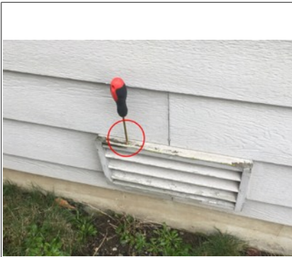
Image of damaged trim on west side of building. Recommend further evaluation/repair by licensed contractor.
