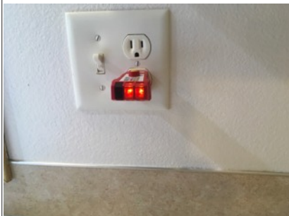
Image of tested GFCI outlet. The GFCI reset is located under the microwave shelf.
