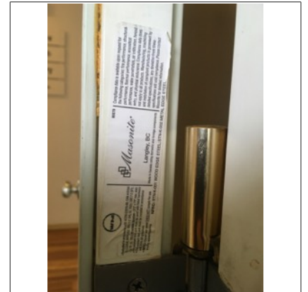
Image of manufacture's tag of the door into/exit from garage.
