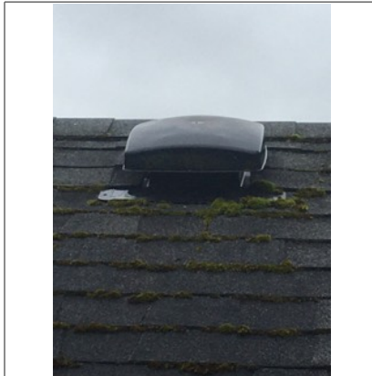
Image of roof venting (multiple vents on roof)
