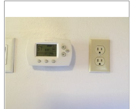
Image of thermostat located in living room.
