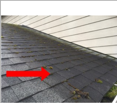
Moss (mold) build-up on roof coverings. Recommend further evaluation by licensed roofing contractor.
