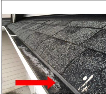
Asphalt shingle granules are evident in gutter system.
