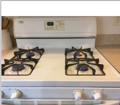
Image of gas stove. All burners operable.
