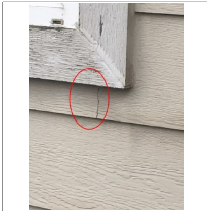
Crack on siding board. Recommend sealing to prevent water intrusion.
