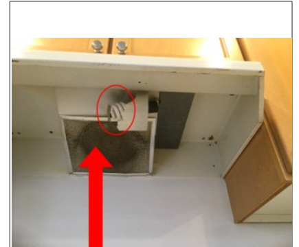
The light bulb cover on the kitchen hood is cracked/damaged. Recommend repair by licensed contractor. The exhaust filter is dirty and should be cleaned.
