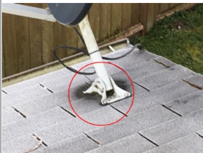
Image of satellite dish on east side of building, Recommend sealing screw holes to prevent water intrusion into roof structure.
