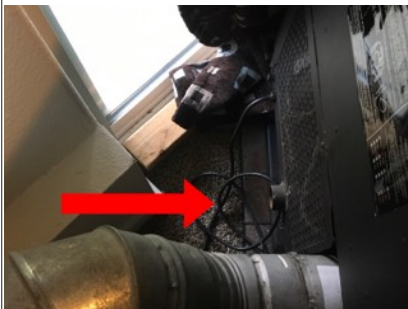
Room heater was not plugged in.
