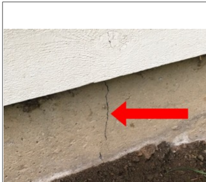
Image of foundation crack on west side of building. This crack does not appear to be structural in nature. Recommend sealing crack to prevent water intrusion.
