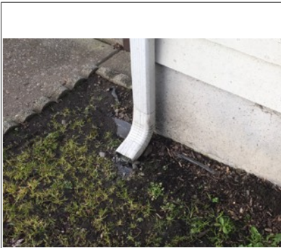
Image of downspout. Downspout may need extension away from structure. Recommend monitoring.
