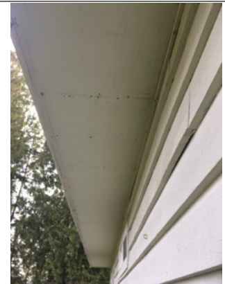
Image of soffit (above 1st story)
