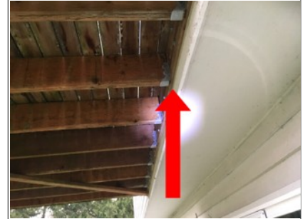
Image of improperly installed caulking under the ledger board. Water that drops down from the top of the ledger board could become trapped by the caulking on the bottom. Recommend further evaluation/repair by licensed contractor.
