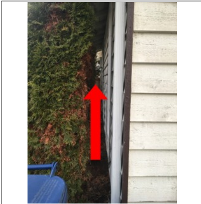
Image of shrubs in close proximity to siding and soffit. Recommend trimming shrubs back to allow for ventilation.
