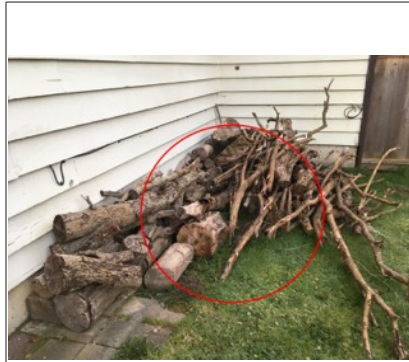
Image of conductive material next to siding/foundation. Recommend moving firewood away from structure to reduce possibility of wood destroying organisms.
