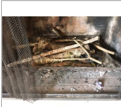
Image of firebricks and fire chamber.
