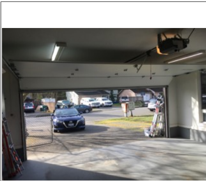
Image of garage door opener operation.
