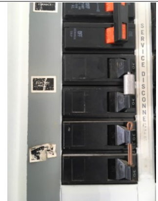
Image of 30 amp breaker in question (hot water tank)
