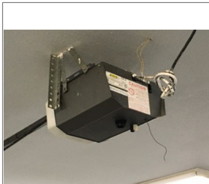
Image of garage door opener
