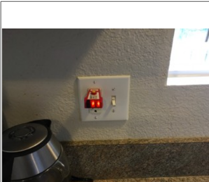
Image of tested GFCI receptacle.
