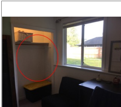
Image of missing closet doors.
