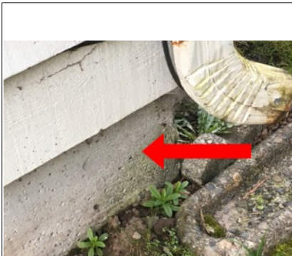
Slight deterioration/pitting of foundation wall around downspouts. Recommend repair of downspout and extend drainpipe away from foundation. Recommend further monitoring of foundation wall.
