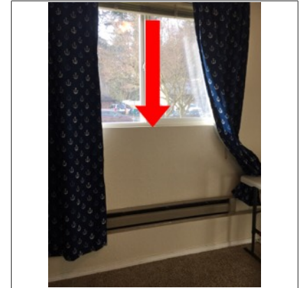
Restricted egress from bedroom due to height of wall (measured from floor to window sill)
