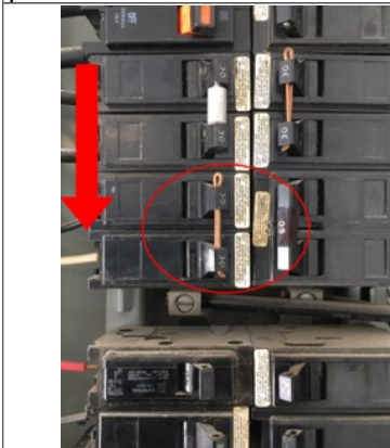
Image of potentially overheating breaker (see thermal image). This breaker has 30 amp supply but conductors appear to be undersized for amps. Recommend further evaluation/repair by licensed electrical contractor.
