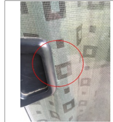
Image of damaged screen on patio door. Recommend replacing screen.
