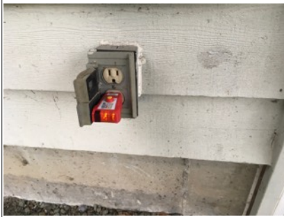
Image of tested exterior electrical receptacle.
