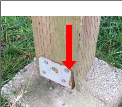
Image of rusted deck post bracket and slight damaged to wood on lower right corner. Recommend further evaluation/repair by licensed contractor.
