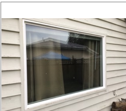
Image of exterior window. Flashing is not installed around exterior windows.
