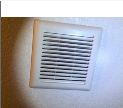
Image of exhaust fan.
