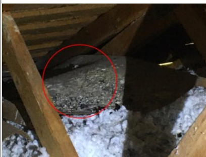
Image of past nesting of birds/animals. Recommend further monitoring.
