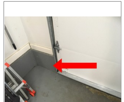
Image of missing eye sensor on door opener. This is a potential SAFETY HAZARD and recommend repair by licensed contractor.
