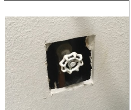
Image of water shutoff valve inside laundry room, next to water heater
