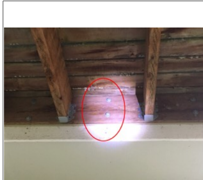
There should be 2" spacing of the fasteners from the ledge board edge and 5" staggered between fasteners. Recommend further evaluation/repair by licensed contractor.
