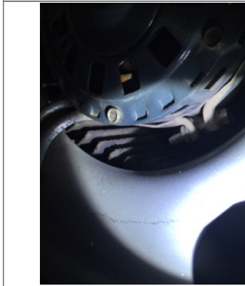
Image of dust on the squirrel cage fan/housing. Recommend cleaning by licensed HVAC contractor.
