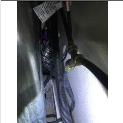
Image of clothes dryer exhaust duct
