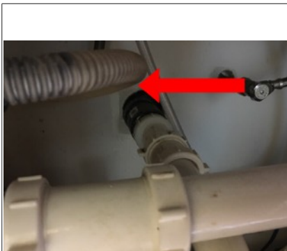
Image of high loop coming from dishwasher. Airgap not installed.
