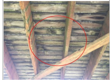
Image of potential wood deterioration of decking surface. Recommend further evaluation/repair by licensed contractor.
