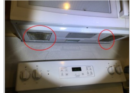
Image of grease filters for exhaust fan. Recommend periodic cleaning to help airflow.
