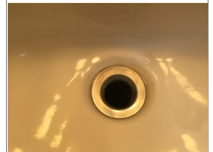
Image of missing sink stopper. Recommend replacement.
