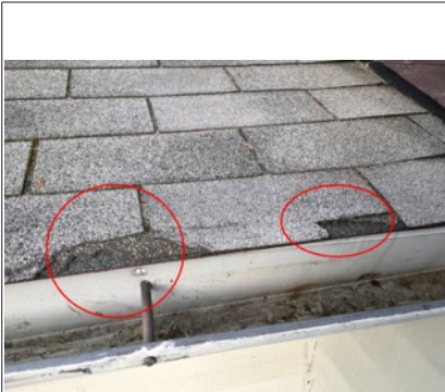
Image of damaged roof shingles near entry door. Recommend further evaluation/repair by licensed roofing contractor.
