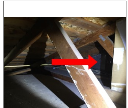
Image of fire separation between garage and dwelling.
