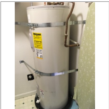
Image of water heater with proper restraints.
