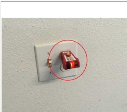
Image of tested electrical receptacle. The outlet on the east side of the garage, near the garage door, has an open ground. Recommend further evaluation/repair by licensed electrical contractor.
