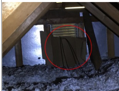
Image of gable vent being blocked by cardboard baffle. Recommend removing cardboard to allow better airflow in attic.
