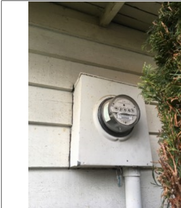
Image of service entrance
