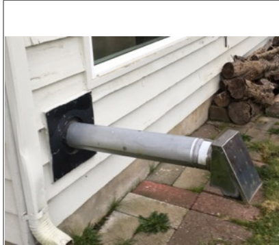
Image of heater exhaust vent outside family room.
