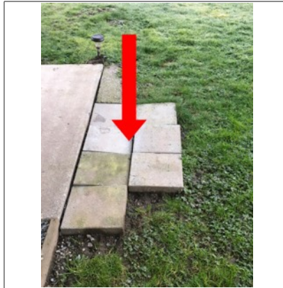
Image of loose and uneven pavers at end of patio. Recommend leveling pavers to reduce trip/fall injury
