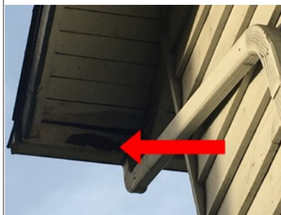
Image of damaged paint on soffit/facia near downspout. Recommend further evaluation/repair by licensed contractor.
