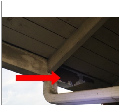
Image of damaged paint on soffit/facia near downspout. Recommend further evaluation/repair by licensed contractor.
