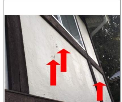
Image of deterioration of paint on several locations on the exterior of the home. Recommend repair by licensed painting contractor. I did not detect wood rot at this location featured in the photograph.
