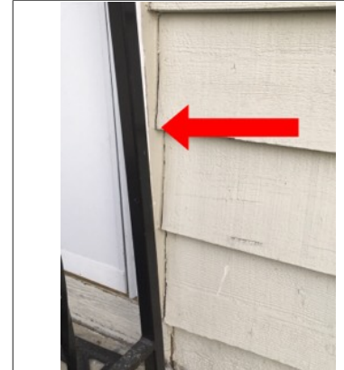
Recommend chasing/sealing around doors, windows, penetrations, and siding joints.
