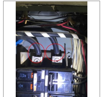
Image of electrical service conductors (stranded aluminum)
