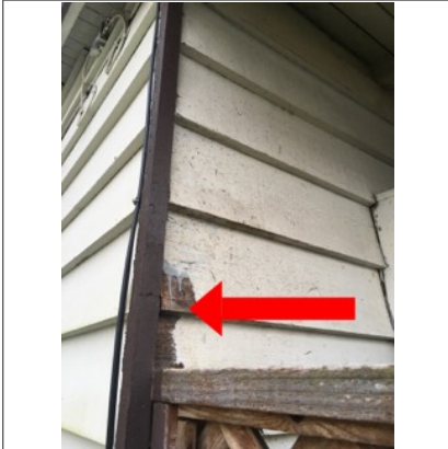
Image of deterioration of paint on several locations on the exterior of the home. Recommend repair by licensed painting contractor. I did not detect wood rot at this location featured in the photograph.
