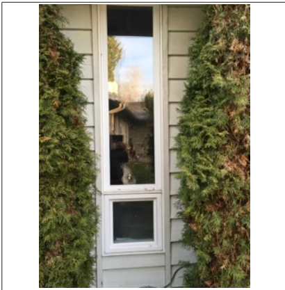
Image of exterior window. Flashing is not installed around exterior windows.
