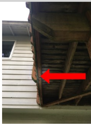
Image of bowed floor joist. Recommend further evaluation/repair by licensed contractor.
