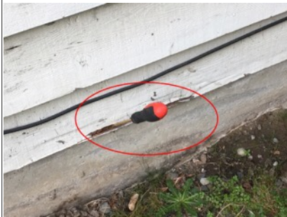
Image of wood rot on west side of building. Recommend repair by licensed contractor.
