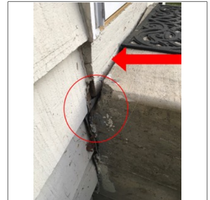
Image of crack at the top of the stairs leading to front door. This crack was probably due to shifting/settling of the stair foundation. Recommend further monitoring.
