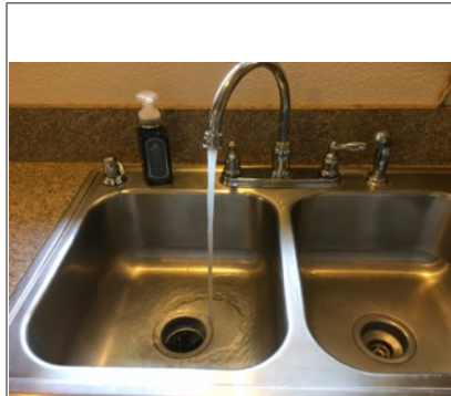
Image of water flow in sink
