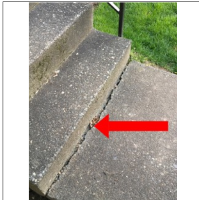
Image of crack at the base of the stairs leading to front door. This crack was probably due to shifting/settling of the stair foundation. Recommend further monitoring.
