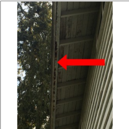
Image of rusted gutters on the south side of the home. Recommend further evaluation/repair by licensed contractor.
