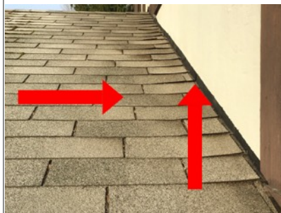
Image of light curling of asphalt shingles on garage roof. Recommend further monitoring.
