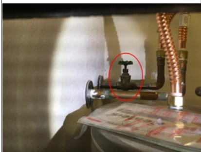
Image of copper pipes and water shutoff valve to hot water tank.
