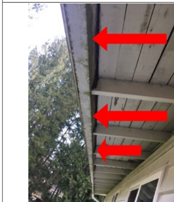
Image of damaged paint on soffit/facia. Recommend further evaluation/repair by licensed contractor.
