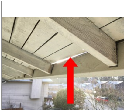
Image of the gutter detaching from the fascia board on the front side of the house. Recommend further evaluation/repair by licensed contractor.
