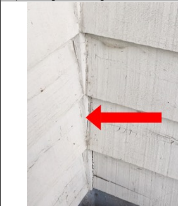
Recommend chasing/sealing around doors, windows, penetrations, and siding joints.
