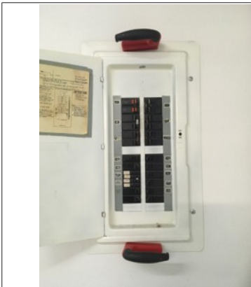
Image of electrical service panel
