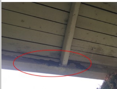
Image of damaged paint on soffit/facia boards. Recommend further evaluation/repair by licensed contractor.
