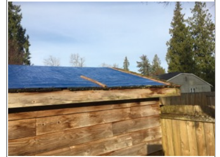
Image of damaged roofing material on shed not evaluated during inspection
