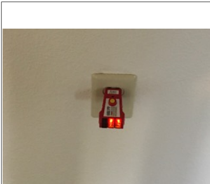
Image of tested electrical outlet.
