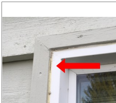
There are several windows on the exterior that will need caulking.
