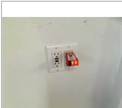
Image of tested GFCI receptacle in garage.
