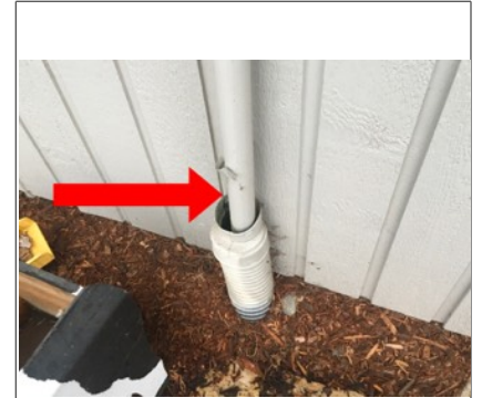
Loose drain pipe bracket.
