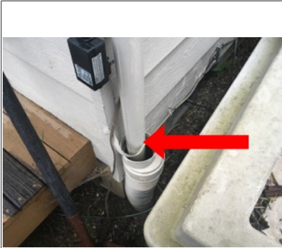
Loose drain pipe bracket.
