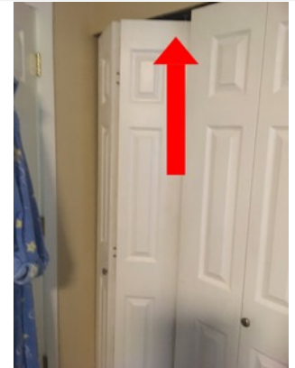
The folding closet door does not properly operate.
