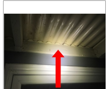
Patio cover should be attached to the structure with lag bolts or screws. Recommend further evaluation/repair by licensed contractor.
