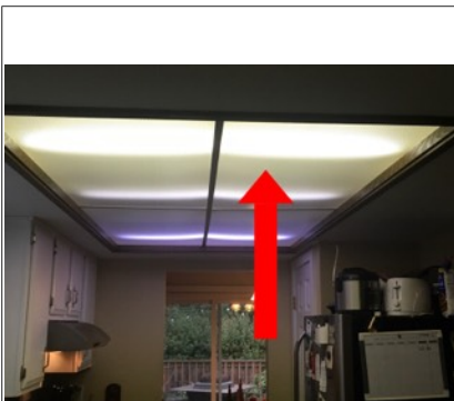
There could be burned out bulbs or lighting ballasts that may not be working. Recommend further evaluation/repair by licensed electrical contractor.
