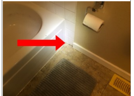
Broken/Missing tile from baseboard in bathroom. Recommend further evaluation/repair from licensed contractor.
