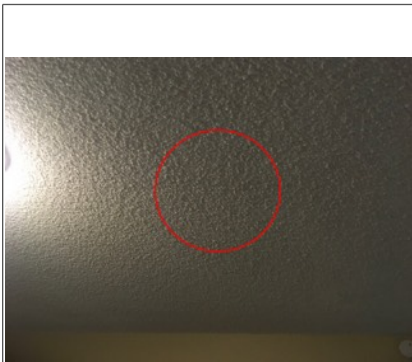
Popcorn ceilings may contain asbestos material.
