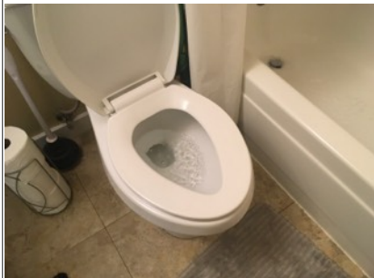
View of water flushing rom toilet.
