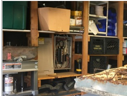
Improper access to electrical panel. Recommend further evaluation/repair by licensed electrical contractor.
