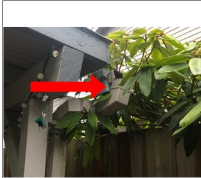
Gutter detached from structure. Recommend further evaluation from licensed roofing contractor.
