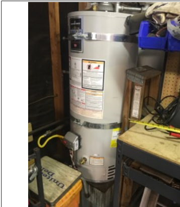
View of water heater with correct seismic straps attached.
