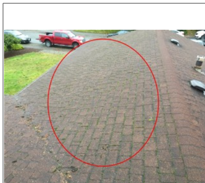
Large portion of roof surface has moss build-up. Recommend further evaluation/repair by licensed roofing contractor.
