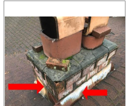
Chimney flashing is rusted and pitted. Recommend further evaluation/repair by licensed chimney specialist.
