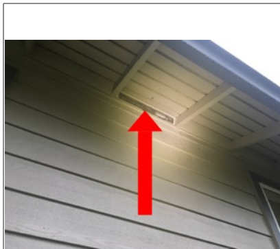
Soffit vent has hole in mesh screen. Recommend further evaluation/repair by licensed contractor.
