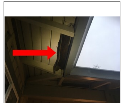
There appears to be moisture penetration into the soffit and fascia boards. Recommend further evaluation/repair by licensed contractor.
