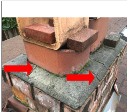
Chimney cap is cracked and could be allowing water penetration into flue. Recommend further evaluation/repair by licensed chimney specialist.
