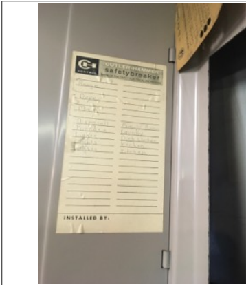
View of breaker data sheet.
