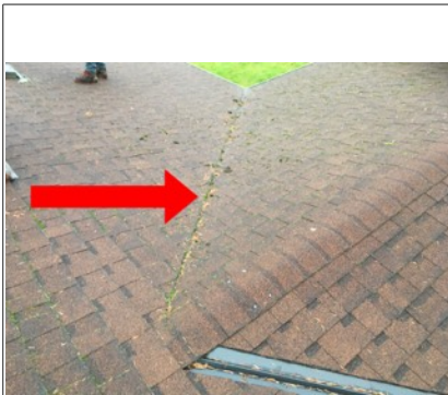
Closed valley that has moss and debris build-up along the valley. Recommend further evaluation/repair by licensed roofing contractor.
