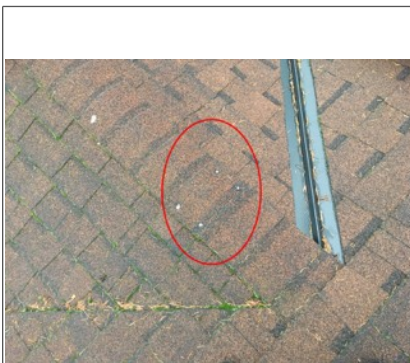
It appear that single repair was improperly completed. Nail holes should be sealed. Recommend further evaluation/repair by licensed roofing contractor.
