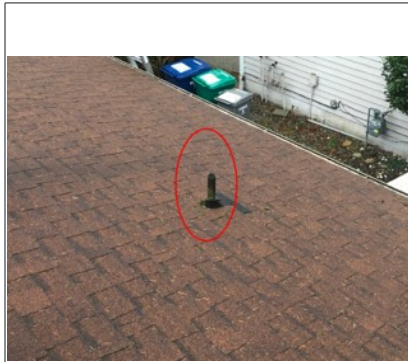
View of plumbing vent
