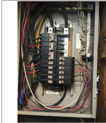
View of inside electrical panel
