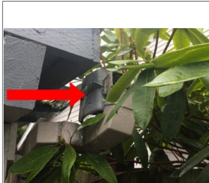
Gutter system has detached from the structure. Recommend further evaluation/repair by licensed contractor.
