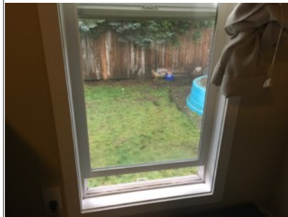
Windows in master bedroom should be installed with safety glass due to lower edge being below 18 inches. Recommend further evaluation/repair from licensed contractor.
