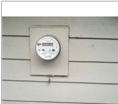
View of service meter
