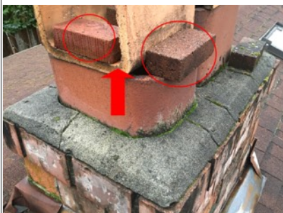
Loose bricks are being used as a rain shield for the chimney flue. This is a SAFETY ISSUE due to restricted airflow from the chimney and potential falling hazard from unsecured bricks. Recommend further evaluation/repair by licensed chimney specialist.
