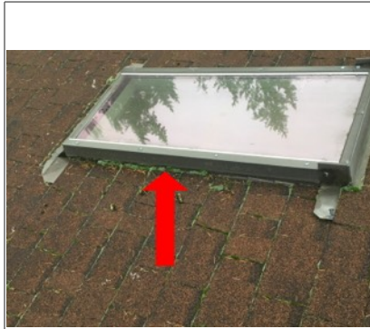
There is moss and debris build-up along flashing. Recommend further evaluation/repair by licensed roofing contractor.
