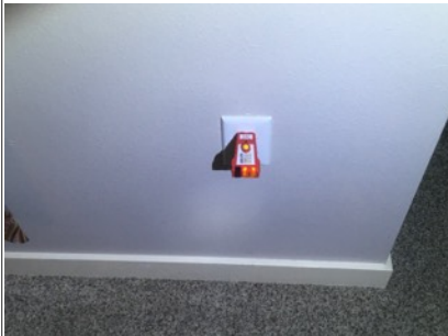
Image of tested outlet in left bedroom
