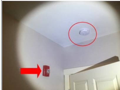
Image of smoke detector in circle in left bedroom. Arrow points to fire alarm that is not tested or inspected and out of scope of home inspection.
