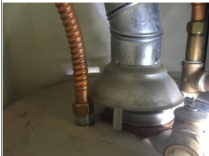
Image of draft hood exhaust for hot water tank
