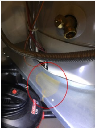
Image of rust from moisture coming from bottom of hot water tank. Recommend further evaluation/repair by licensed plumbing contractor.
