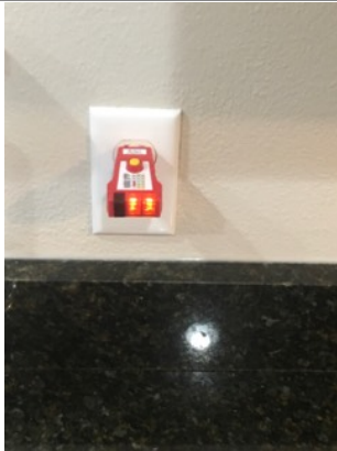
View of GCFI receptacle in the kitchen
