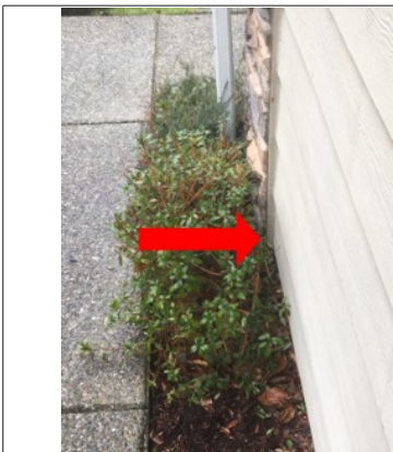
Ground cover in contact with siding recommend trimming vegetation.
