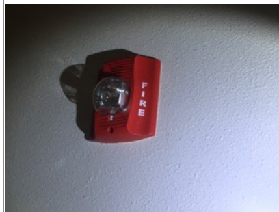
Image of fire alarm. Not inspected or tested-out of scope of home inspection.
