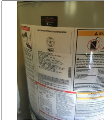
Image of data plate on a hot water tank
