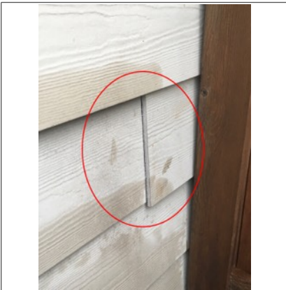
There are several loose boards on the back of the residence.
