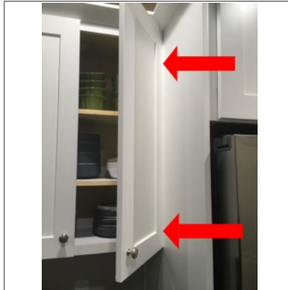
Cabinet is binding on right side against cabinet wall. Recommend adjusting cabinet door or repair by licensed contractor.
