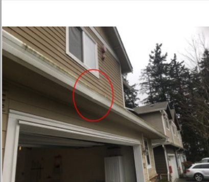
Small dent on front gutter system. This does not effect the functionality of the drainage system.
