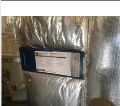
Image of HVAC filter door
