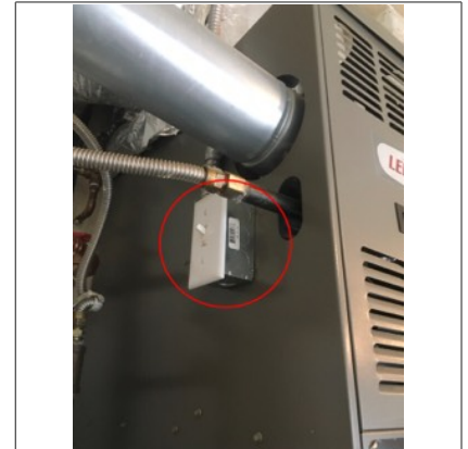
Image of electrical shut off for HVAC
