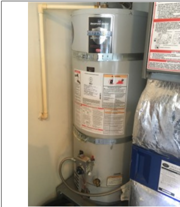
Image of hot water tank
