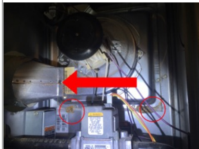
Image of condensation buildup inside HVAC unit. Recommend repair/evaluation by licensed HVAC contractor.
