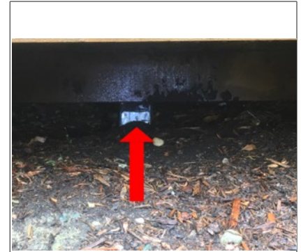
Deck post and joist bracket in contact with soil. Recommended remove soil from around post.
