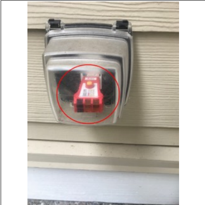
Exterior GCFI outlet not functional and could not be tested. Recommend further evaluation/repair by qualified electrical contractor.
