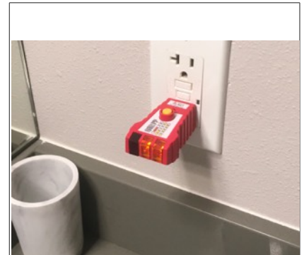
Image of tested GCFI receptacle in bathroom. This GCFI outlet is upstream of both first story bathrooms.
