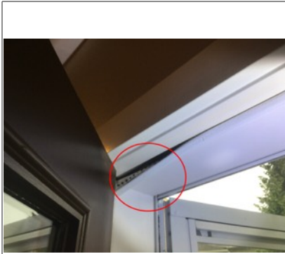
Weather stripping loose on back door (to deck). Recommend further evaluation/repair by licensed contractor.
