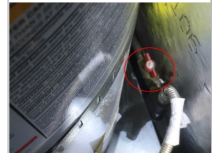
Image of gas shut off valve for hot water tank
