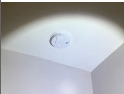
Image of smoke detector in right bedroom
