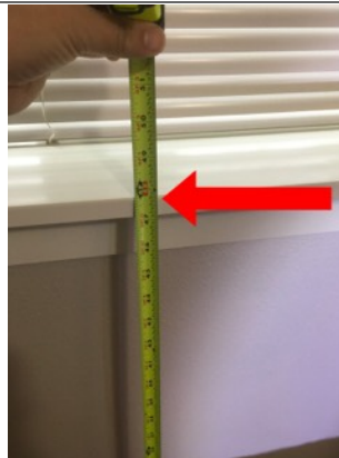
Master bedroom window is 47 inches above floor and for safe egress should be 44 inches. This could potentially be a safety issue and recommend further evaluation by licensed contractor.
