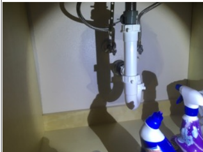
Image of plumbing under left sink.
