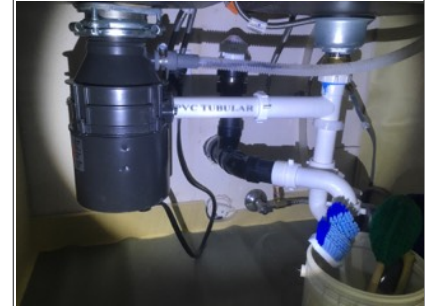
View of plumbing under kitchen sink
