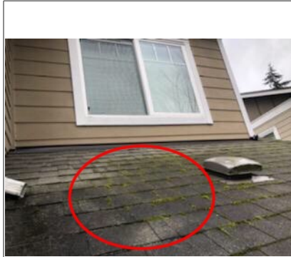
Image of moss build-up on asphalt shingles. Recommend cleaning by licensed roofing contractor.
