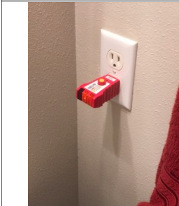
Image of GCFI receptacle in bathroom
