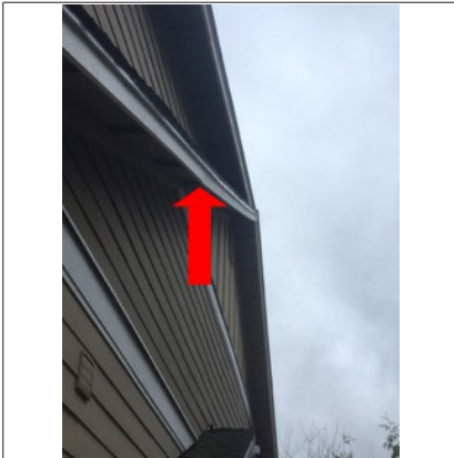
Fascia board on side of building is twisting/separating from supports. Recommend further evaluation/repair by licensed roofing contractor.
