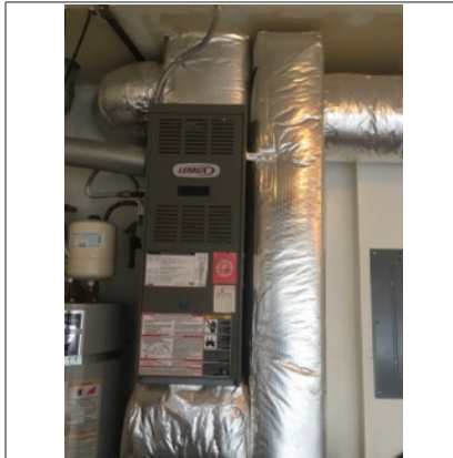
Image of furnace located in garage
