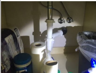
Image of plumbing on the left sink in master bath
