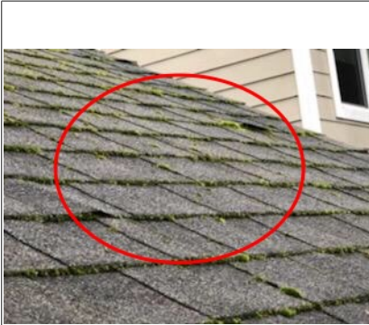
Image of moss build-up on asphalt shingles. Recommend cleaning by licensed roofing contractor.
