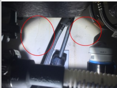
View of stains on back of cabinet/wall under kitchen sink. There was no visible leak. Stains could be from damaged grout/sealing of backsplash and counter.
