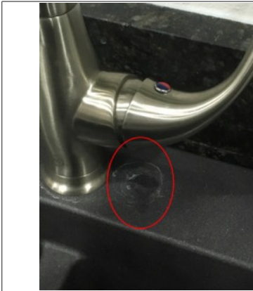
Visible water leak coming front handle on sink. There was a small circle on counter under handle indicating ongoing leak. Recommend further evaluation or repair by licensed plumbing contractor.
