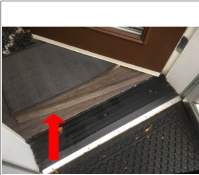
Back door threshold is loose and not properly installed. Recommend further evaluation/repair by licensed contractor.
