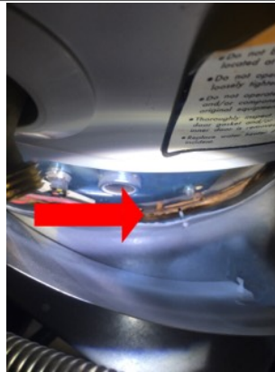
Image of rust on the bottom of the hot water tank. Recommend further evaluation/repair by licensed plumbing contractor.
